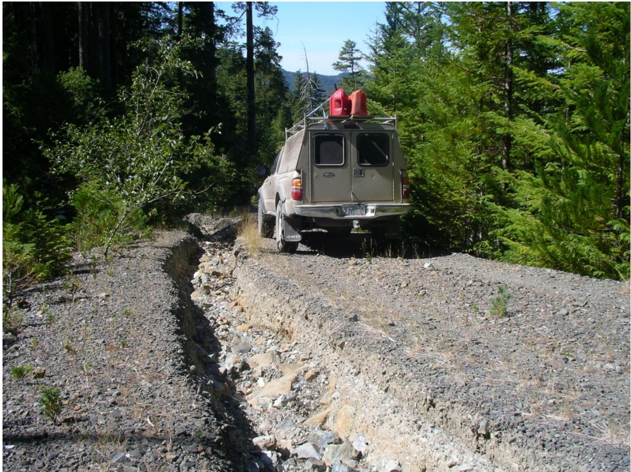
FSR3237130: Lack of routine maintenance such as ditch cleaning and road grading may prevent water from leaving the road prism, which can result in gullies and/or slides that contribute sediment to the stream network and increase costs.
