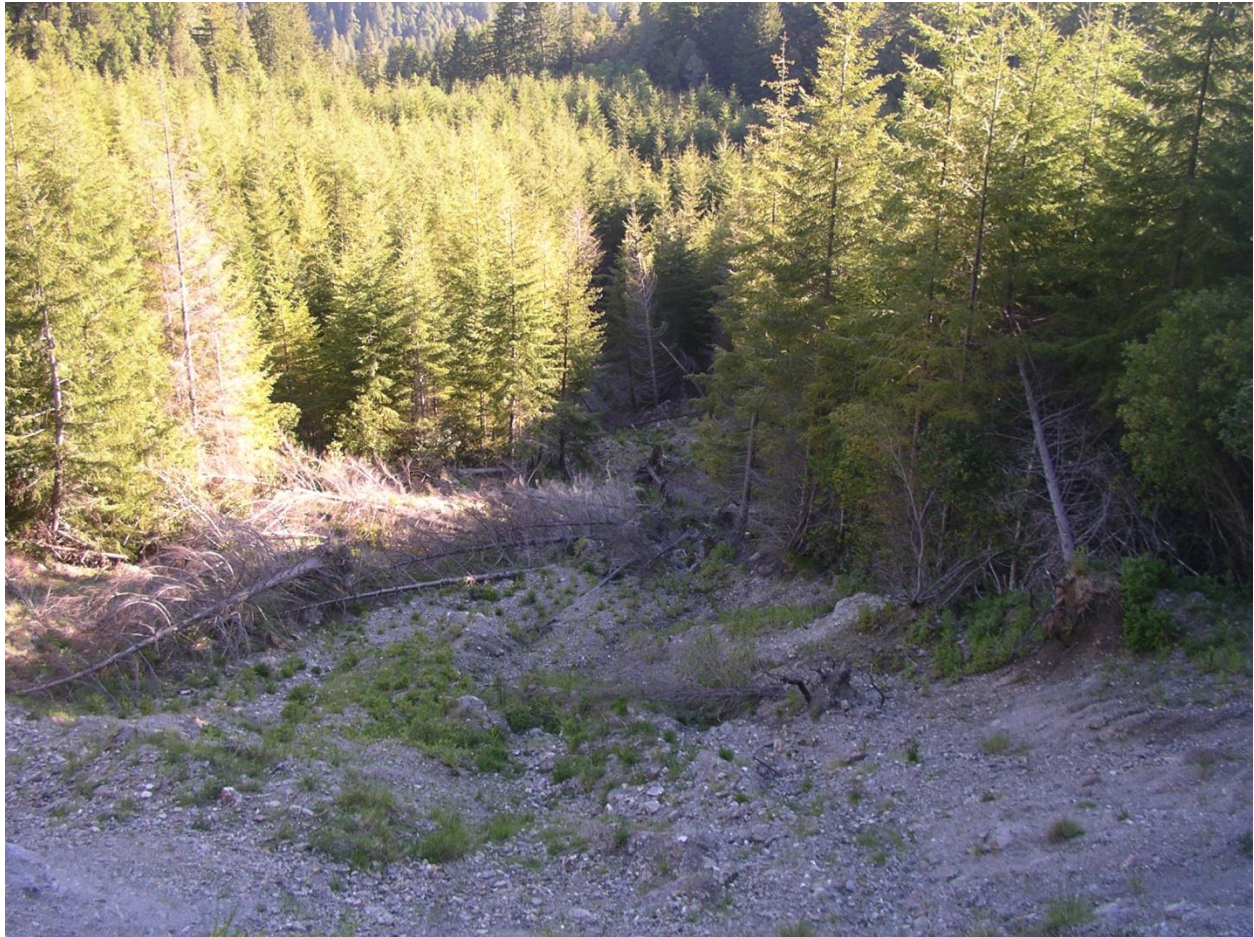
FSR3340140: Road fills displaying cracks, scarps, and/or horsetails are at risk of failure. In Lobster Creek these failures have potential to “run-out”, which destroys forest and timber resources and may contribute sediment to the stream network. Reconstruction often requires realignment, which can be a significant, if not prohibitive, expense.
